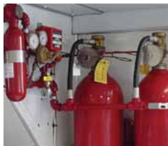
Total Flooding CO 2 System
